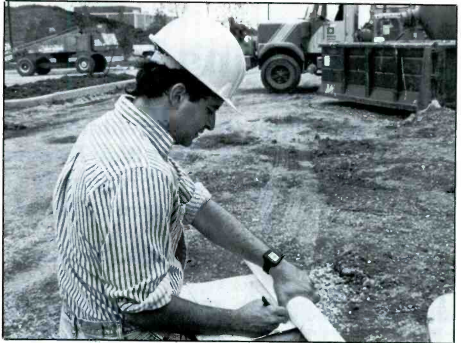
This construction foreman is wearing a new Motorola pager that looks like a wristwatch.
